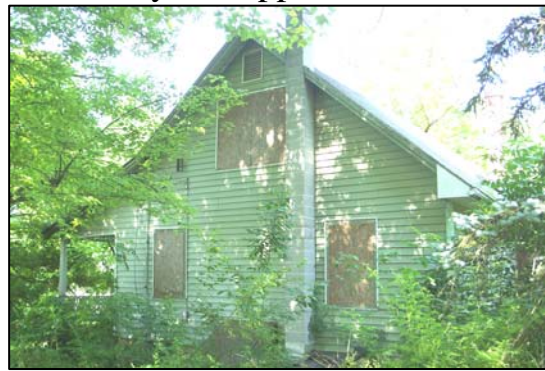
118 Creamery Road - Tax Id#: 28-06-072.0300 1½ Story House in Very Poor Condition on 1.1 Acre Lot with On-Site Well & Septic Total 2017 Taxes: $3,505
